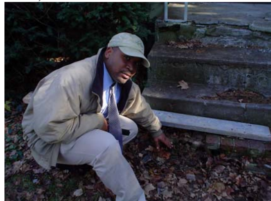
ASHI CERTIFIED Inspector Mel Wilkes points out damaged brick to a client on an inspection.
