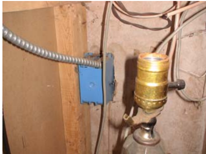
Metal clad wire installed in a plastic box.
