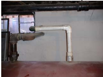
Oil tank breather made out of PVC plastic
