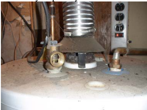
No extension pipe on relief valve and wrong duct material for chimney on a gas water heater.
