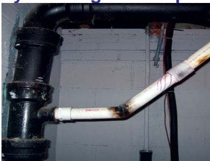
Homeowner Plumbing...we'll make it bend with a torch... from John Cranor Cranor Inspections Glen Allen, Va.
